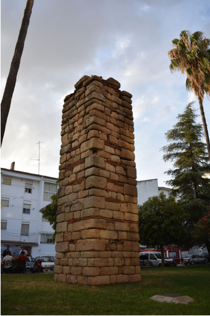
Fig. 2 Failed sixth-century repair of a pillar of the Los Milagros aqueduct, Mérida
