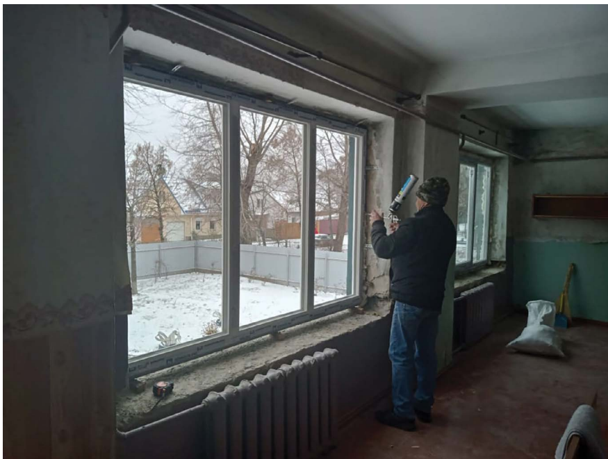
Figure 2.4 Local buildings are repaired and renovated for temporary accommodation in Ukraine. (Photograph by K. Adalgeirsdóttir)
