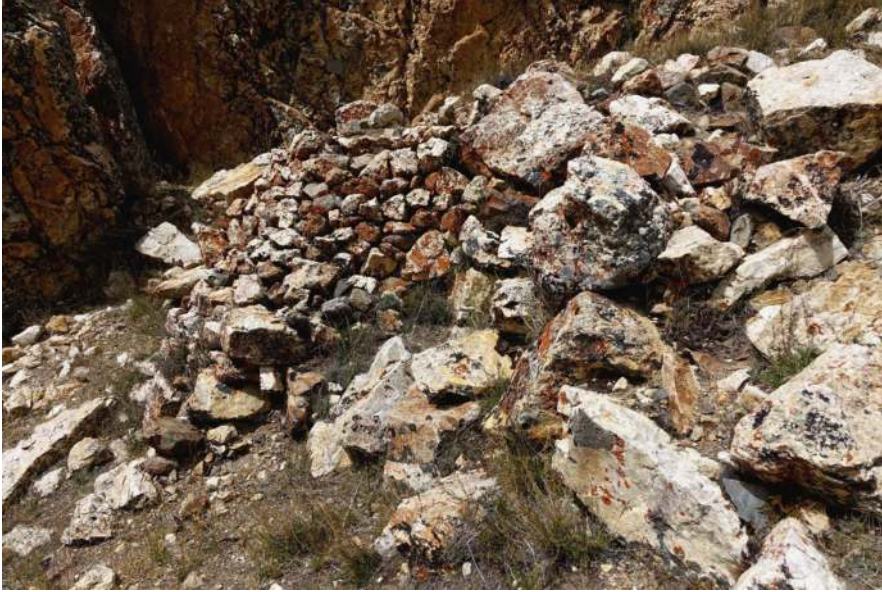
Figure 56. The lone structure at the bottom of the upper complex, a highly degraded revetment. This was part of a more extensive structure at one time. Note the orange lichen covering the stones of the wall.
