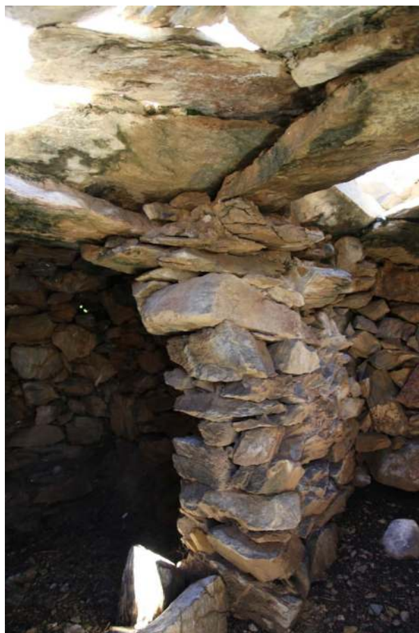
Figure 102. A wall buttress in the house in the summit sector, Do dril bu. Note how many corbels and bridging stones converge on this wall for support. After so many centuries this arrangement now seems rather precarious.
