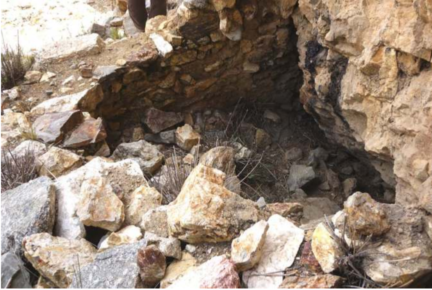
Figure 75. The semi-subterranean room built into a recess in the formation of the lower tier. The remnants of the series of corbelling that once encircled the top of the walls are visible.
