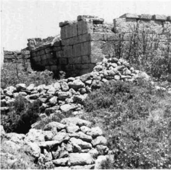
Illus. 263. Mtaugat: the church, masonry leaning outwards in need of buttressing.
