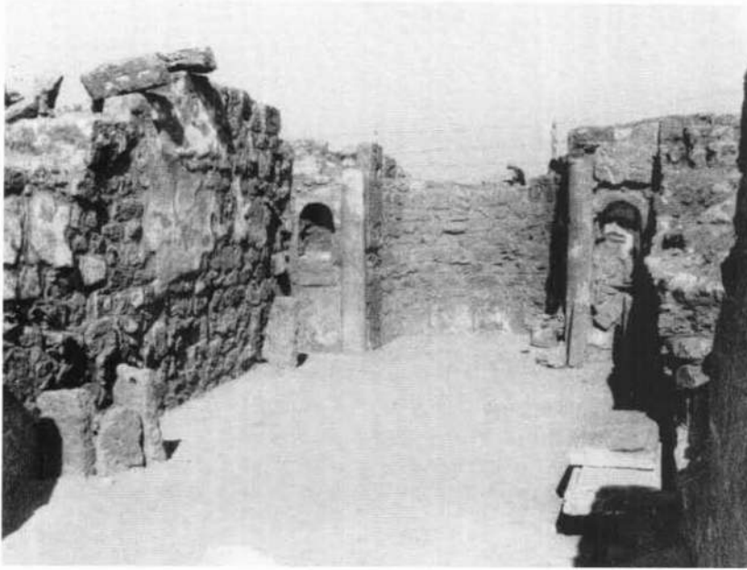
Illus. 32. Apollonia/Sozusa: Central Church, south aisle with added apse and niches, a martyrium(?).
