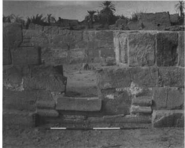
Figure 17.4. Detail of masonry of one of the central buildings at Old Jarma (GER 1.1).
