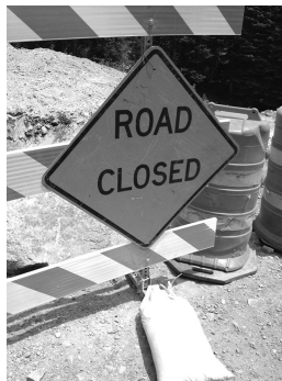
Figure 8.1 Roadblocks come in many forms.
