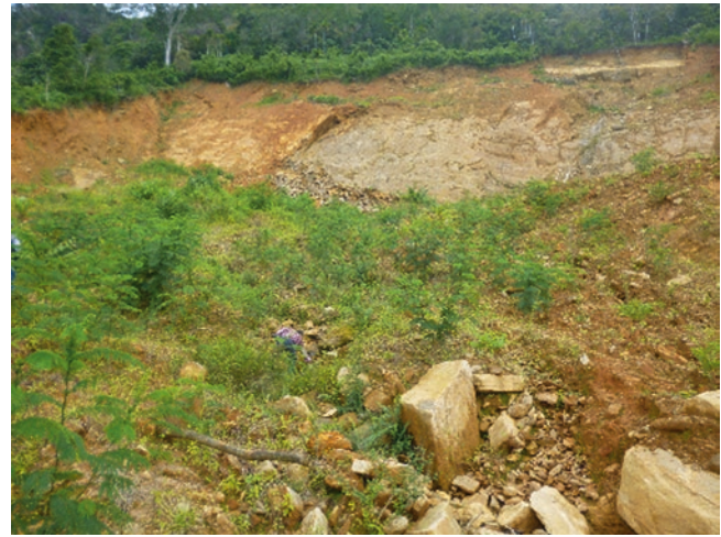
Fig. 4 Close-up view of the crown of the Aranayaka landslide and rock and rock detachment along the foliation joint (Photo by Dias, A.A.V., July 2017)
