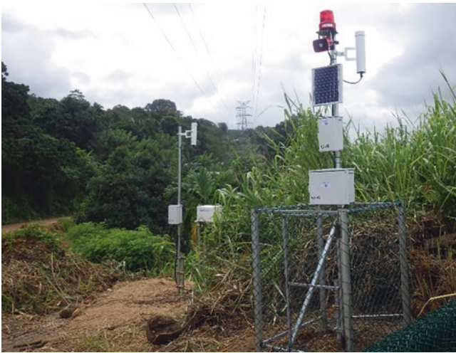
Fig. A.42 Compact alarm device to alert local people to landslide risk
