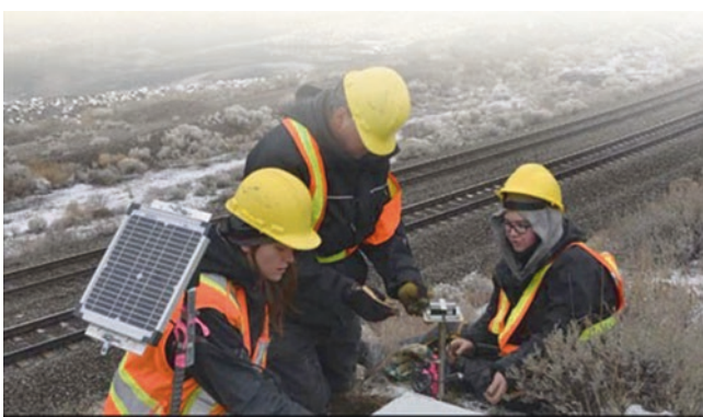
Fig. A.5 The GSC conducts geohazard studies to reduce risks to people and infrastructure, here installing equipment to monitor landslide activity above a critical railway corridor in central BC
