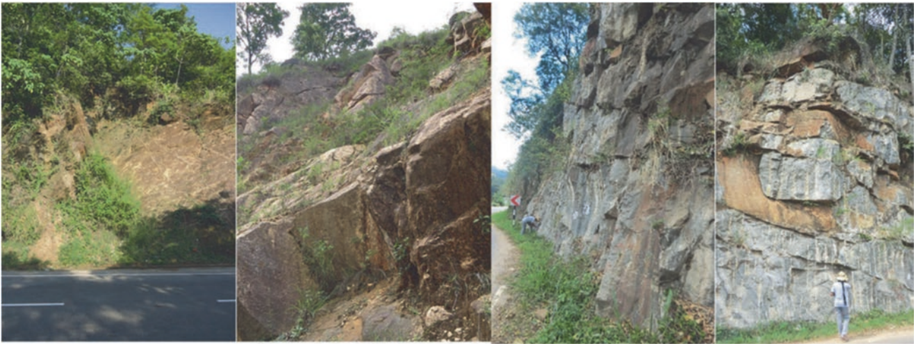
Fig. 30 Example of rock formed failures along the road side slope. Wedge failure, translational slides and falling rocks are very much significant along the road sides. High hazard potential zone can be observed due to foliated and jointed rock formations (Fig. 13 in Dias et al. 2023)
