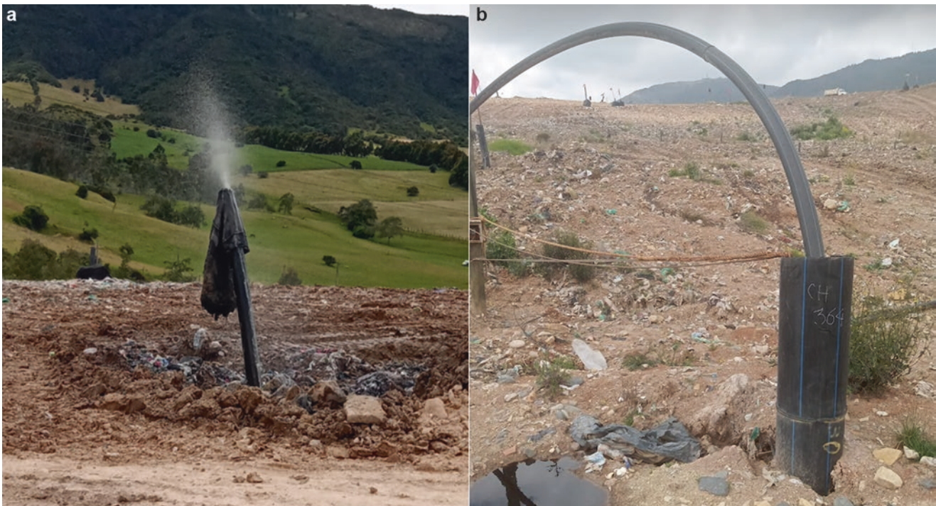
Fig. 5 (a) Pressurized output of leachate through chimneys, (b) chimneys with extraction of leachate by pumping output of leachate through chimneys
