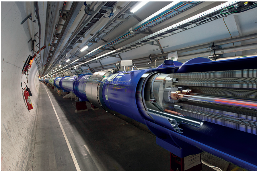
Figure 1.3 LHC dipole magnets in the underground LHC tunnel
