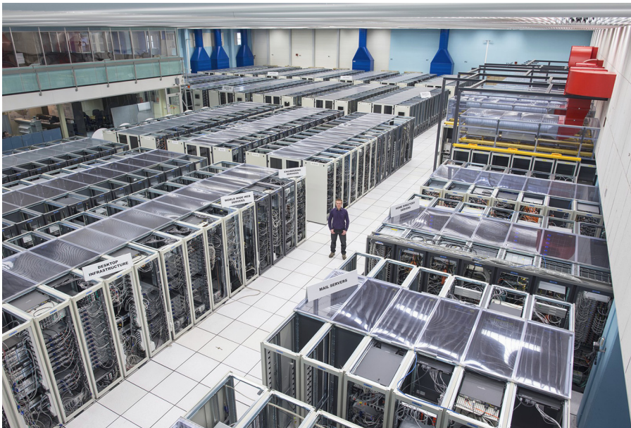
Figure 11.2 CERN's Computing Centre
