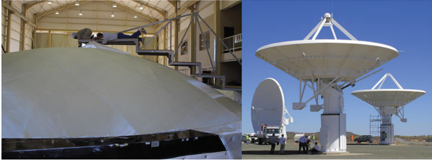
Fig. 6.13 The KAT-7 fibreglass dishes under construction in the Karoo district of South Africa in 2009. Right: The completed KAT-7 dishes being installed in 2009 on what is now the site for MeerKAT and SKA1-Mid
