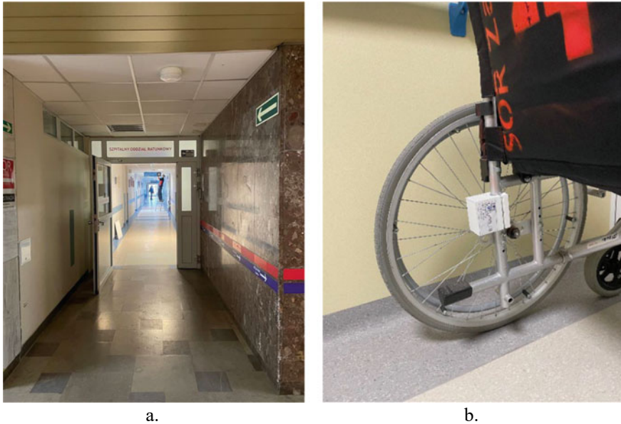
Fig. 7 Test installation of the system in St. Adalbert's Hospital in Gdansk, Poland. a ESPAR antenna installed on the ceiling, b localized device attached to a mobile asset (wheelchair)
