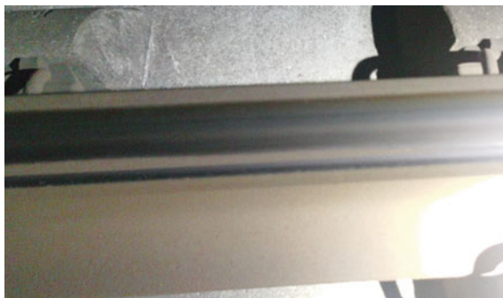
Fig. 3 Rail surface state
