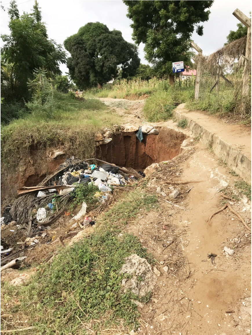
FIGURE 5. A path damaged by rain in Salasala. Photo by author, June 2018.
