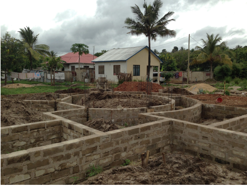
FIGURE 8. An elaborate floor plan with circular living room takes shape on a building site among more modest houses. Photo by author, April 2016.
