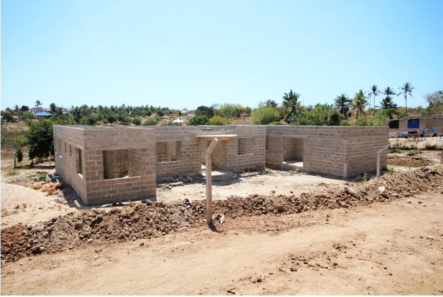
FIGURE 1. A house in the early stages of construction, Salasala, September 2012. Photo by author.
