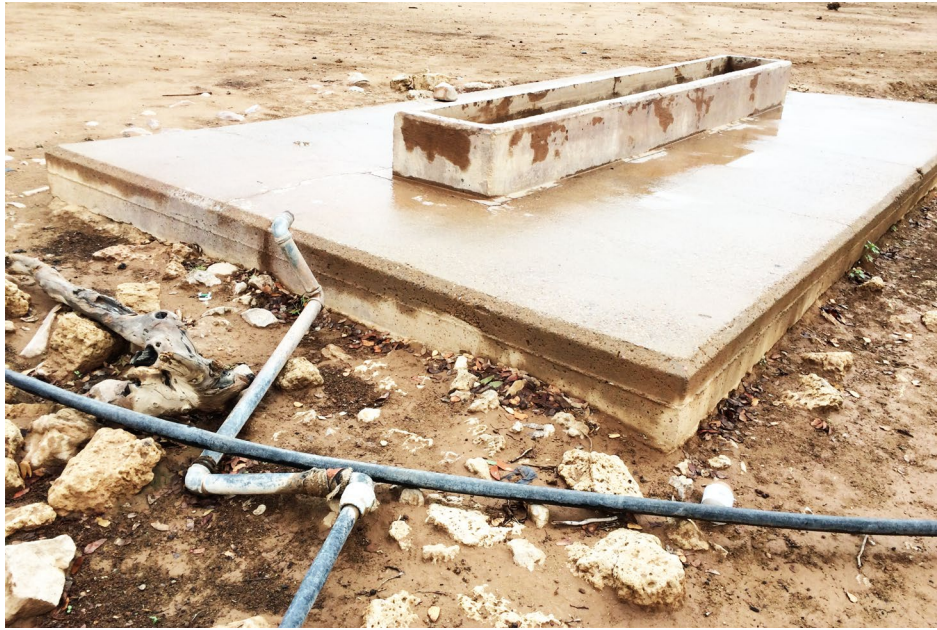
Fig. 11.8 Pipework damage by elephants at the water point in Okazorongua village, Orupupa Conservancy. Photo: © Michael Wenborn, 1.4.2021, CC BY-NC-ND 4.0.
