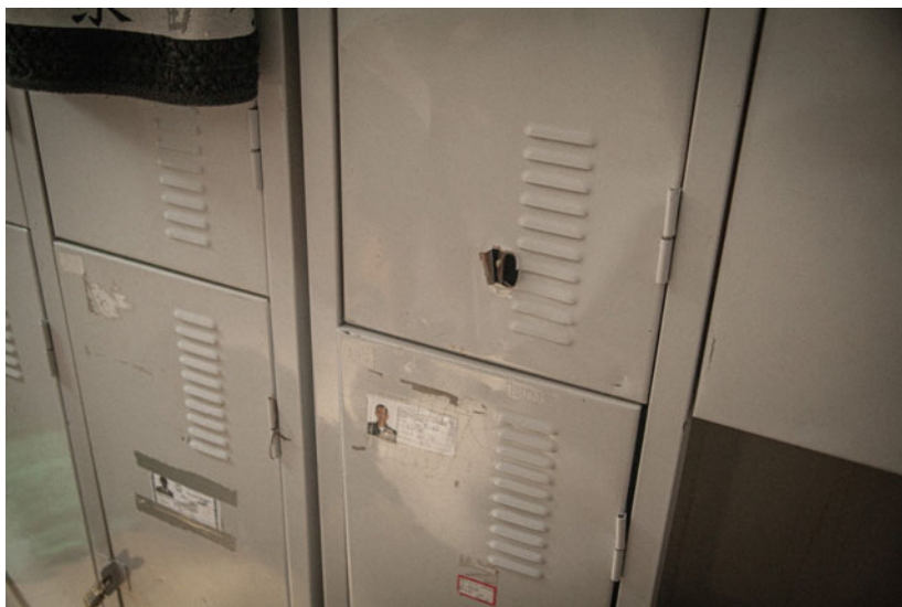
Fig. 4.5 A bullet hole in one of the cabinets at the police officers' resting quarters
