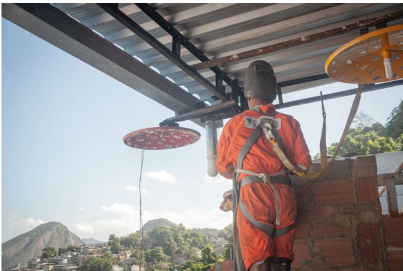
Fig. 2.4 Beto installing the lamps he made with old satellite dishes on a terrace in the favela
