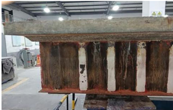
Fig. 3 Uniform corrosion of the web
