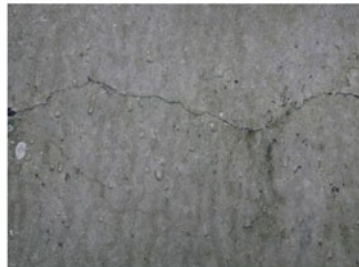
f. Detailed Image of Cracks inside the Tunnel
