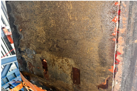
Fig. 4 Uniform corrosion of the base plate
