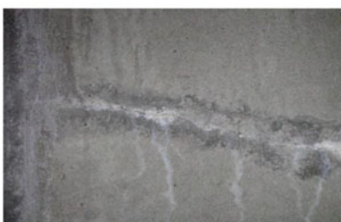
h. Detailed Image of Calcium Analysis of Wall Cracks
