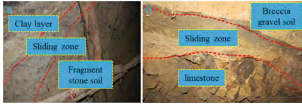
Fig. 4. Characteristics of the sliding belt (a. PD1702 at 26 m on the right wall; b. PD144 at 90 m at the adit).
