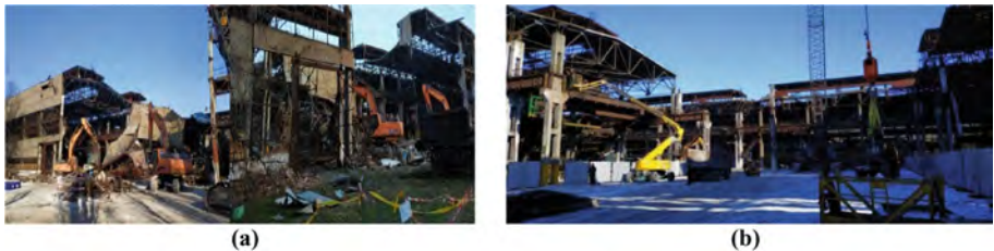
Fig. 4. a. Clearing the site from the demolished structures (photo before), b. Photo of the site after clearing.
