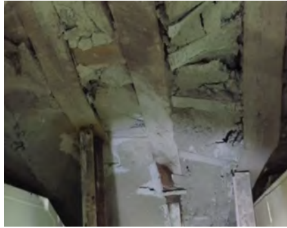
Fig. 2. Soft rock tunnel deformation causing distortion of steel arch frames.
