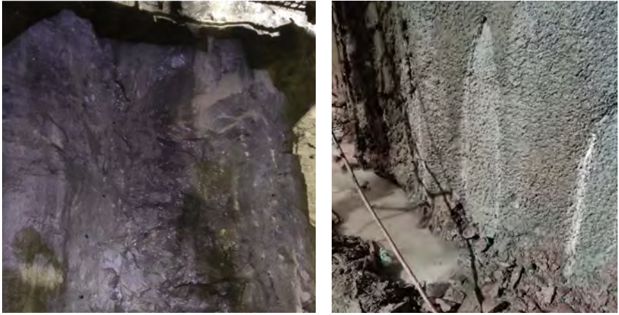
(a) water seepage and gushing from the tunnel face (b) Water surges in the sidewalls of the tunnel
