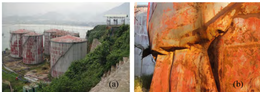
Fig. 1. The aviation fuel depot in Lien Chieu, Da Nang.
