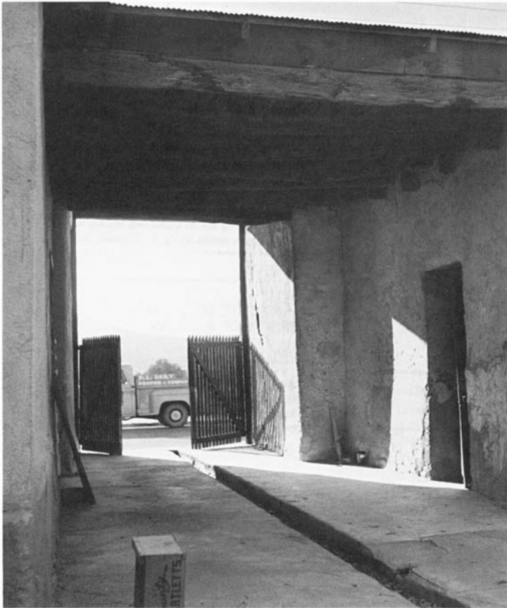
Figure 2.8. Ceiling over the zahuan entrance. (Arizona State Museum photo by James E. Ayres.)
