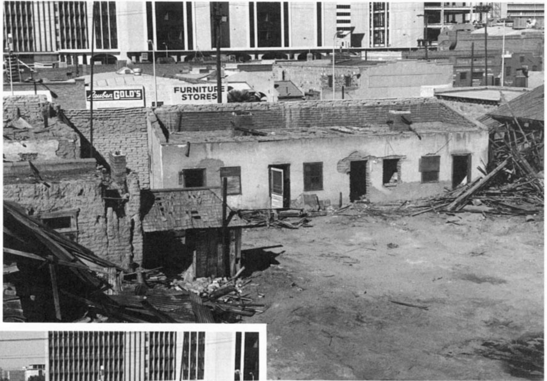
Figure 2.32. A 1968 view north across the Ying On compound patio shows demolition under way: left , the remains of the west wing (Unit 2), with the attached shingle-roofed latrine that once had been the hiding place for emptied containers of illegal opium; center , the four-room north wing (Unit 3); right , one of the last utilized Chinese dwelling rooms; and center right , a corner of the east wing (Unit 4). The low buildings in the background also were removed to make way for a new civic center. (Arizona State Museum photo by James E. Ayres.)
