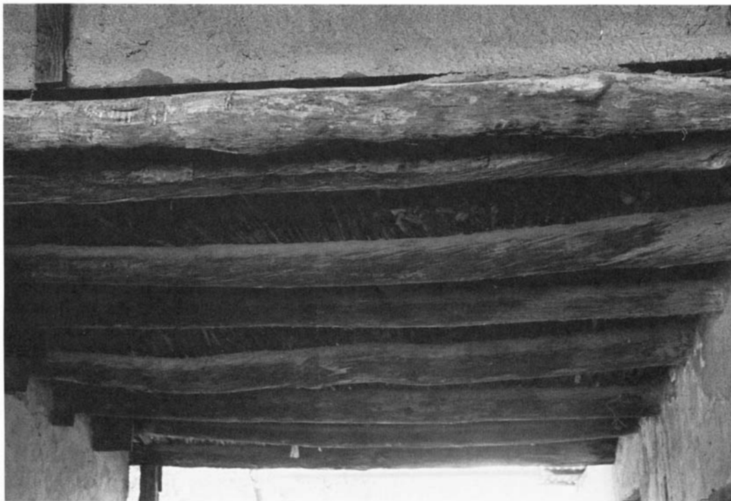
Figure 2.9. Zahuan ceiling construction of pine beams topped with saguaro crossribs and earth, characteristic of most barrio edifices. (Arizona State Museum photo by James E. Ayres.)
