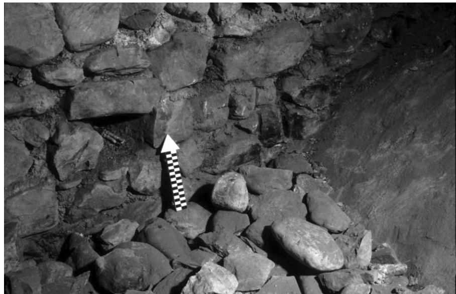
Fig. 2. Chur, cathedral of Assumption, restoration 2001-2007, example of a finding spot in the central roof (© Archaeological Service of the canton of Grisons).
