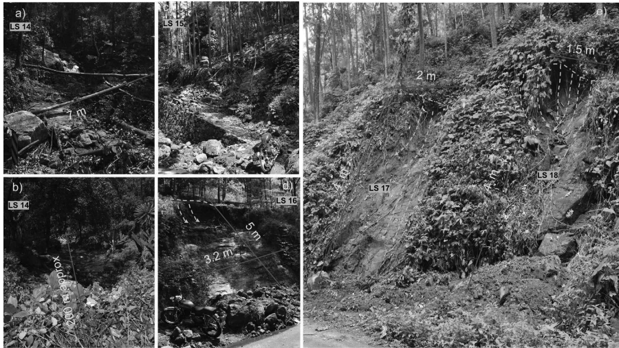
FIGURE 18.5 Landslides at locations 14 to 18: (a) LS 14—runout path above road level, (b) LS 14—runout path below road level, (c) LS 15, (d) LS 16 and (e) LS 17, LS 18.
