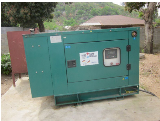
Fig. 9 Backup generator, Sierra Leone. (Photo: Dan Littlefield)
