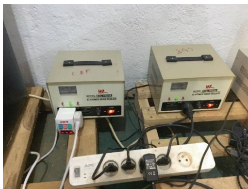
Fig. 10 Voltage regulators mounted on pallets in case of standing water in the building. (Photo: Dan Littlefield)
