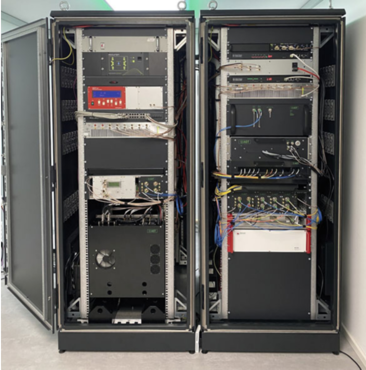
Fig. 8 A photograph of the MARMOT system which is a 19"-rack-mounted room-temperature quantum computer, having a less than 2\text{ m}^2 footprint and a power consumption of less than 2 kW. Designed for the installation at HPC infrastructures and data centers, the PINE setup is located behind a front plate on the bottom of the left rack, while the full laser system and stabilization is placed in the right rack
