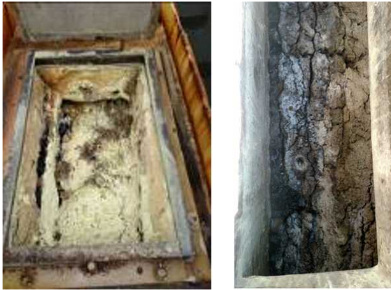
Figure 2.6 Thick and solidified scum layer inside different GLS separators of UASB reactors treating sewage (without proper removal devices and operational routines). Source: Chernicharo and Bressani-Ribeiro (2019).
