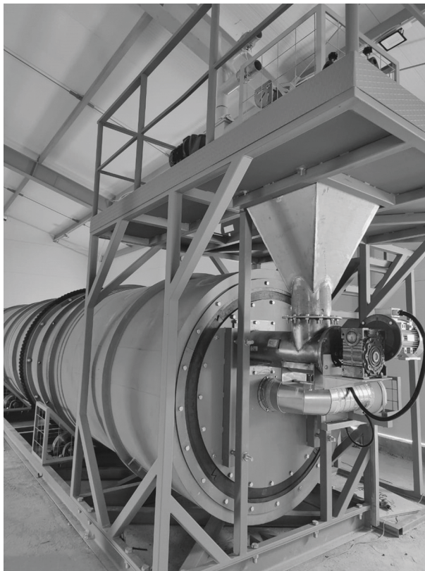
FIGURE 2.7 Automated bio-fermenters for solid organic waste processing.
