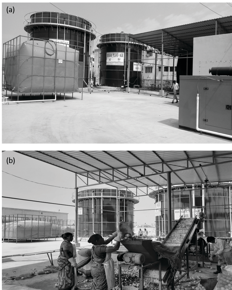
FIGURE 3.3 The 10 TPD biogas plant for the generation of biogas and bio manure from market and vegetable waste at Bowenpally in Telangana State.
