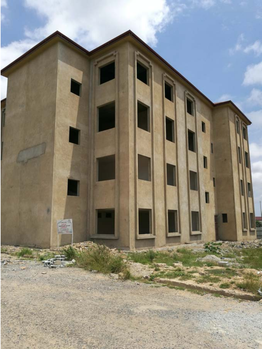
FIGURE 22 Qatar Charity/Aldiaa educational project. Construction of dormitories at (then) Madina Institute of Science and Technology, now Lakeside University College PHOTO: HOLGER WEISS/2017
