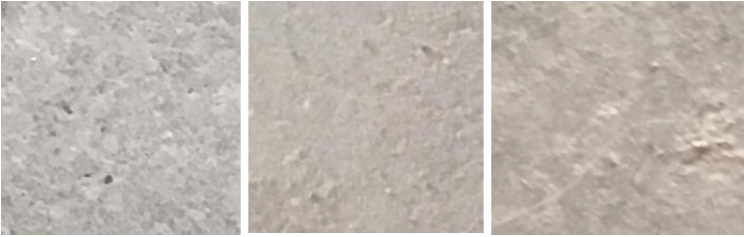
Fig. 3 The intact crack image of dam
