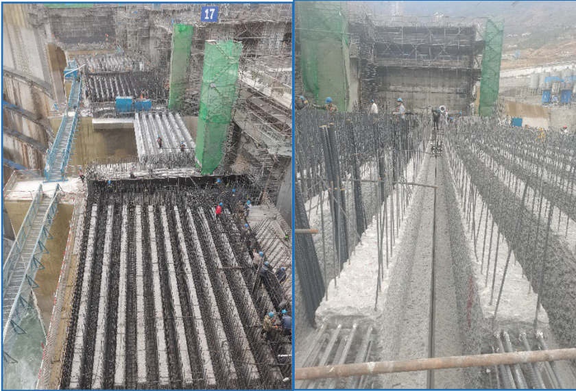
Fig. 17. Installation and construction of inverted “T” - shaped concrete prefabricated beam with table hole support and articulation
