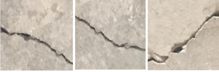
Fig. 4 The crack image of dam
