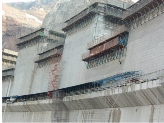
Fig. 9. Downstream hydraulic climbing formwork
