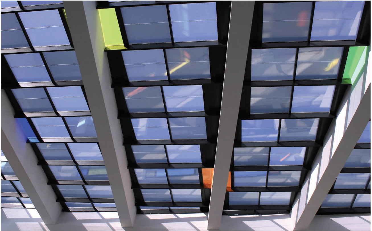
Figure 2.5 Retrofit of a skylight made of semi-transparent a-Si BIPV modules, in the historic Béjar Market in Salamanca, Spain. Photo credits: Onyx Solar.
