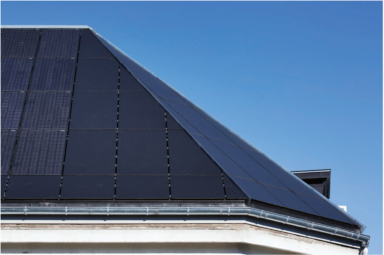
Figure 5.32 Close-up of the BIPV roof at Andreas Bjørns St.1. Credits: Dorte Krogh.
