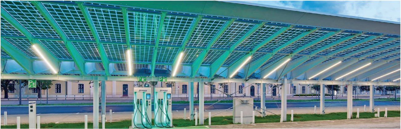
Figure 5.137 Night view of the BIPV car canopy at Schönbrunn. Credits: Ertex solar.
