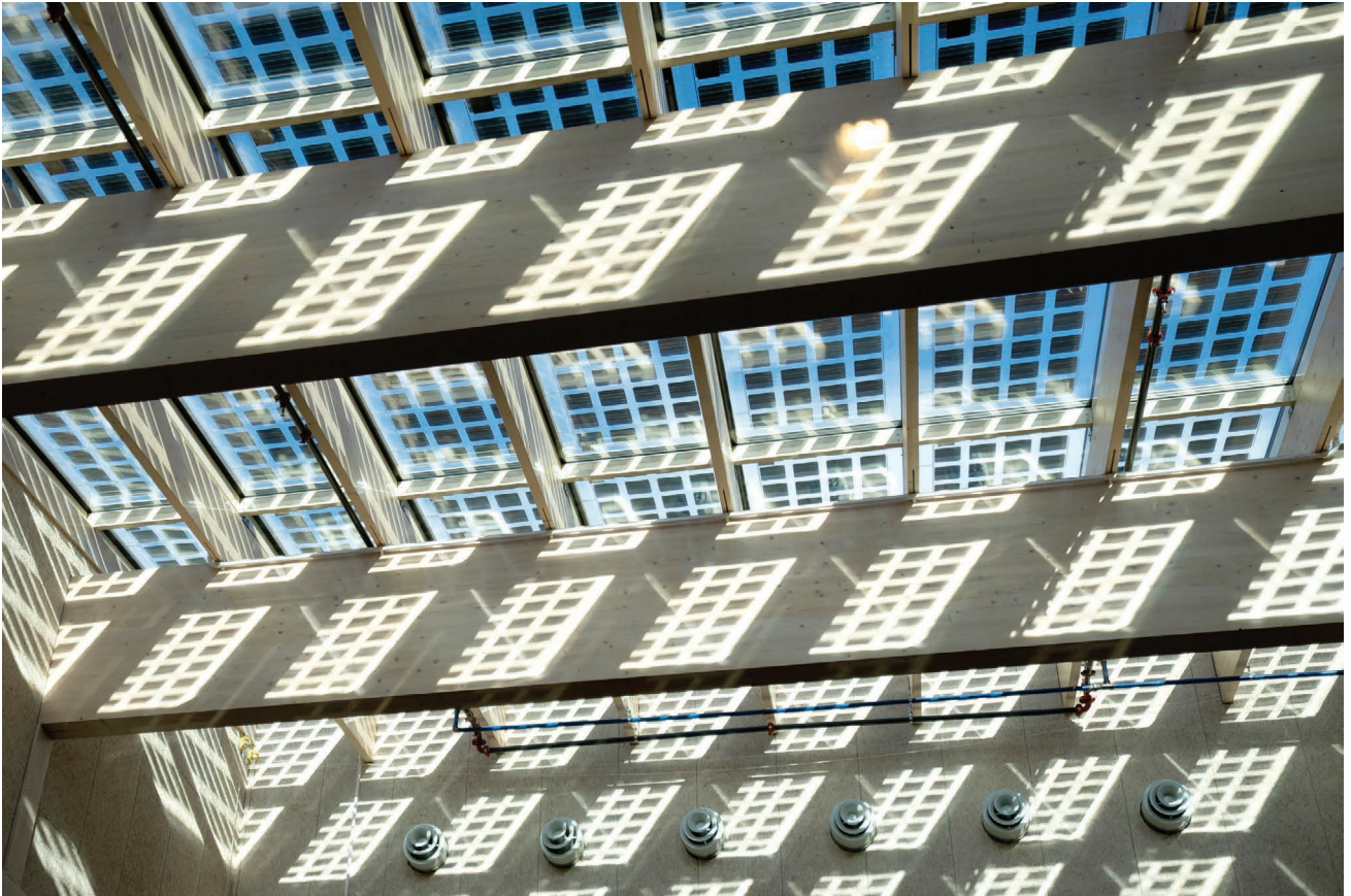
Figure 3.9 BIPV skylight application using insulated glazing with lower cells density for daylight transmittance at the “house of choice” designed by White Architects in Stockholm.
