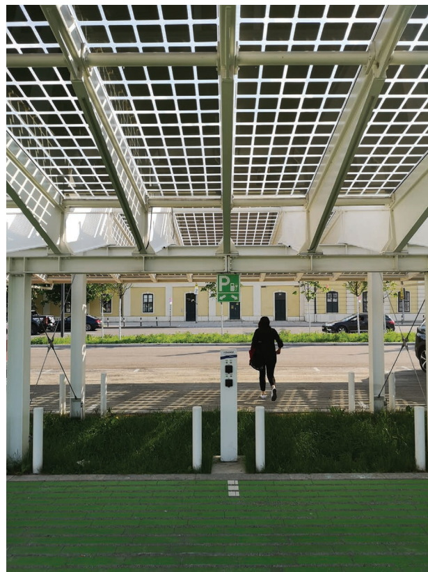
Figure 5.136 Close-up view of the BIPV car canopy at the arrival centre in Schönbrunn. Credits: Francesco Frontini, SUPSI.
