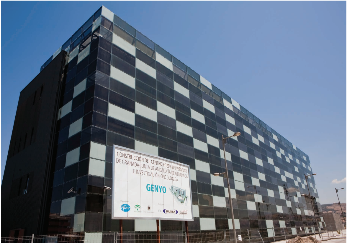
Figure 5.95 Pedestrian view of the Genyo Research facility, showing the BIPV south and west façades under construction. Credits: Onyx Solar.
