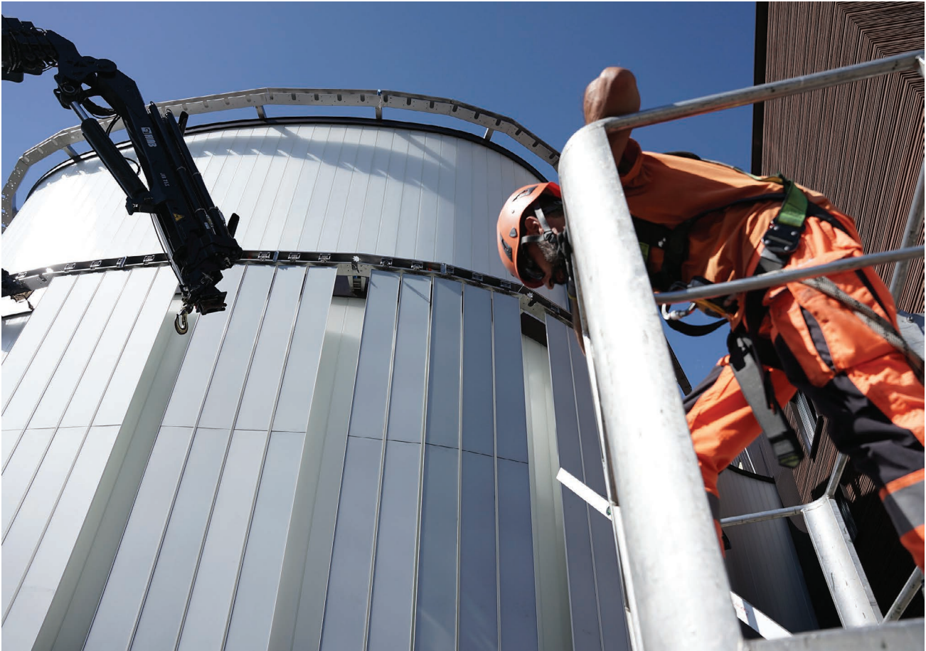
Figure 5.130 Installation of the white movable BIPV solar shading louvres. Credits: Franklin University.
