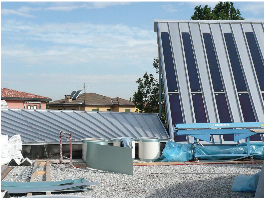
Figure 5.16 Close up of Folzano Kindergarten BIPV roof. Credits: Jennifer Adami, EURAC.
