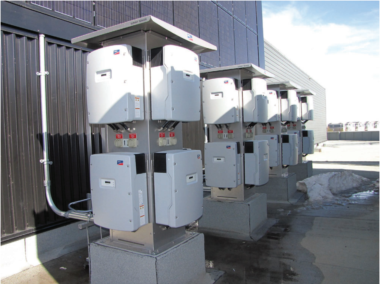
Figure 5.69 Rooftop string inverters at Jeanne & Peter Lougheed Performing Arts Centre. Credits: Credits: Gordon Howell, HME.
