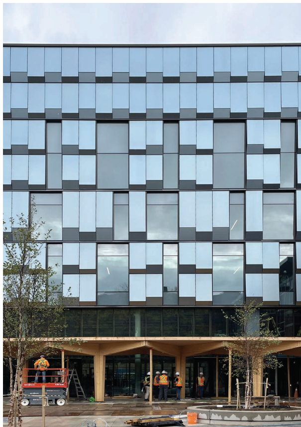
Figure 5.90 Close-up of the Fanshawe College Innovation Village BIPV rainscreen. Credits: Diamond Schmitt Architects.
