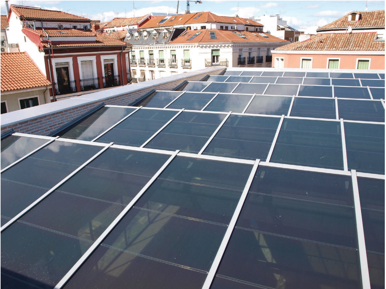
Figure 5.44 Exterior view of the BIPV skylight at San Antón Market. Credits: Onyx Solar.
