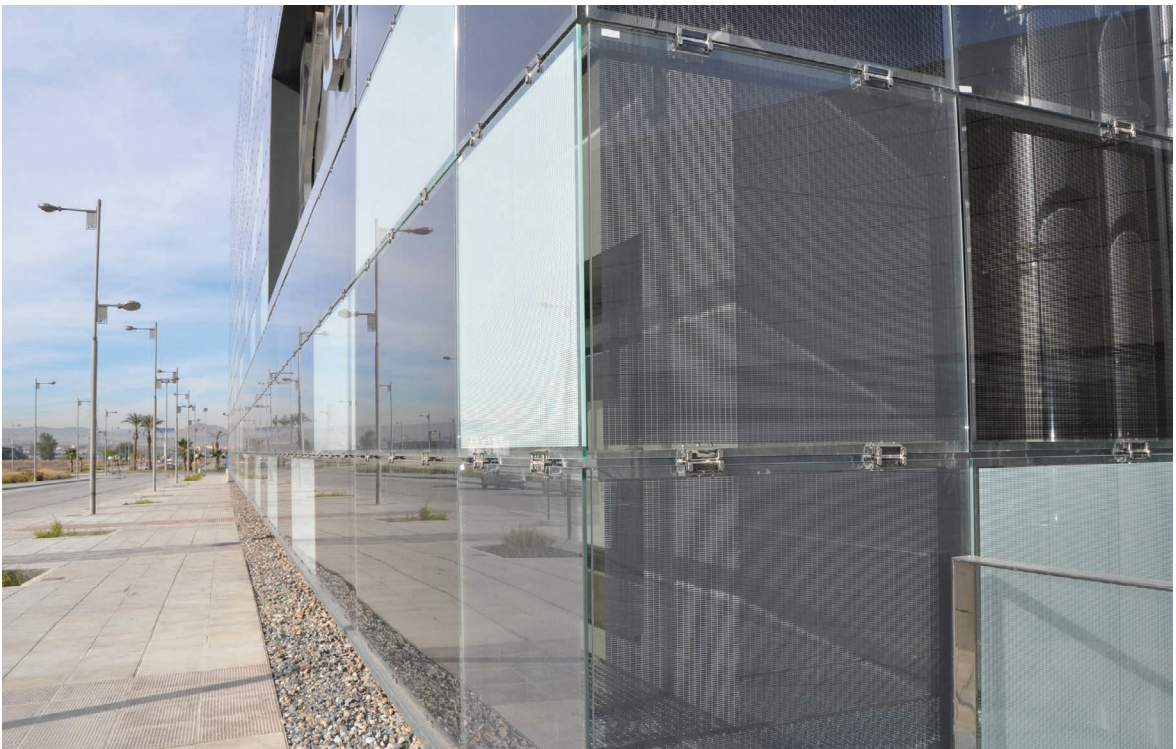
Figure 5.96 Detail of the BIPV double skin façade of the Genyo Research facility. Credits: Onyx Solar.
