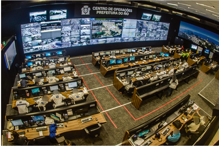
Fig. 11.2 Rio de Janeiro operation center's control room. Source: Author's personal archive (2016)
