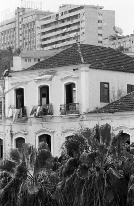
Figure 1.2. Palácio Dona Ana Maria Joaquina, prior to reconstruction in 1992. Source: John Liebenberg.
