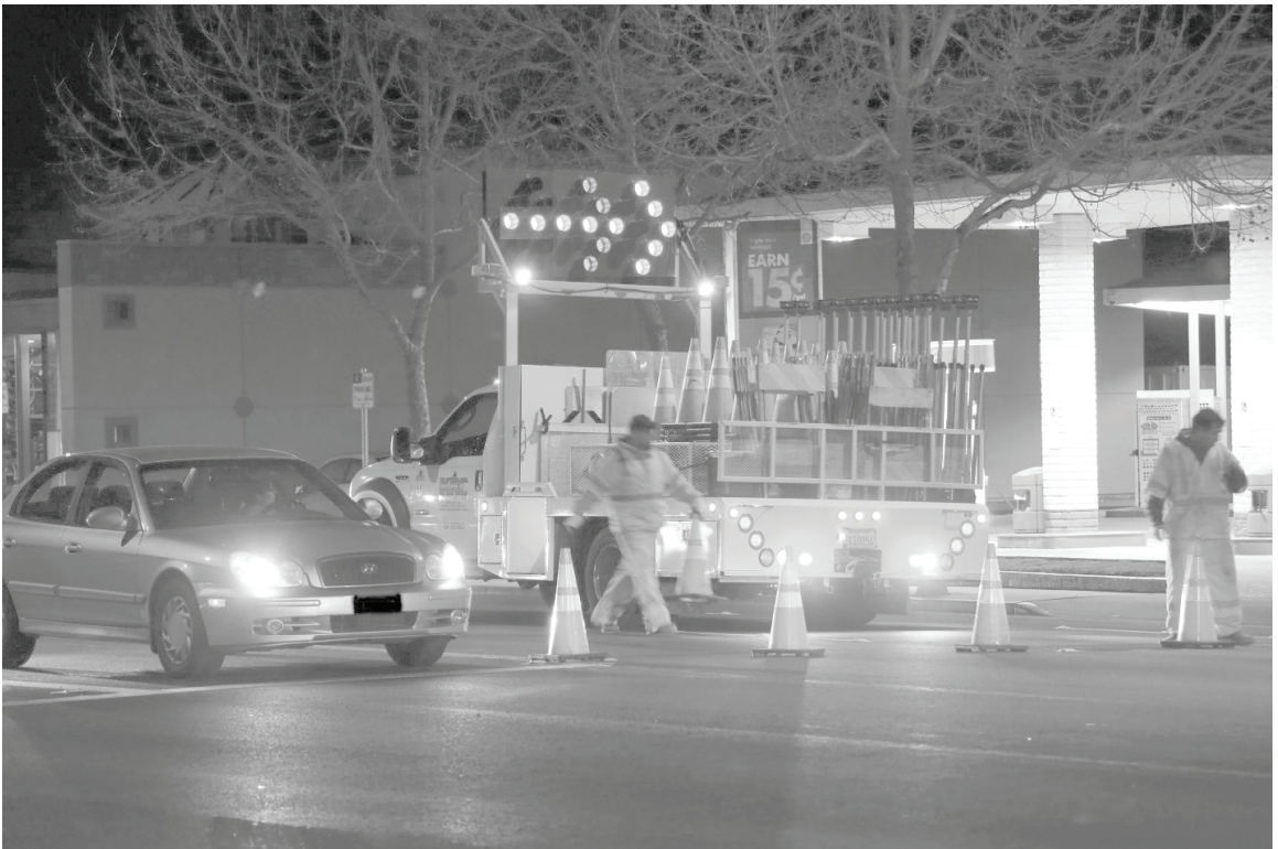
Figure 11-6. Traffic control and the use of reflectorized vests at a utility construction site.
