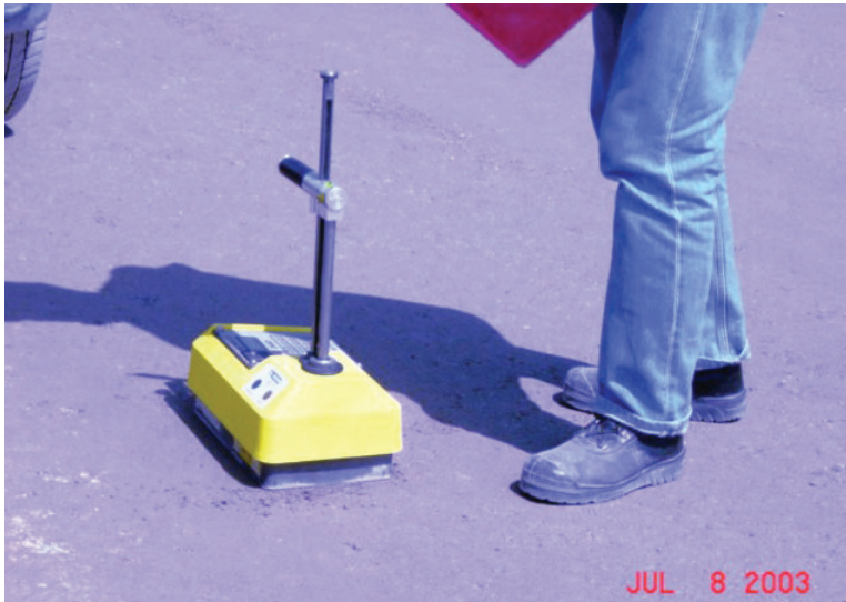
Figure 6-23. Measuring compacted soil density with a nuclear gauge. These devices can measure asphalt density as well as the soil moisture content. The project specifications will direct the required frequency of density testing, often per lift or per volume of compacted soil.
