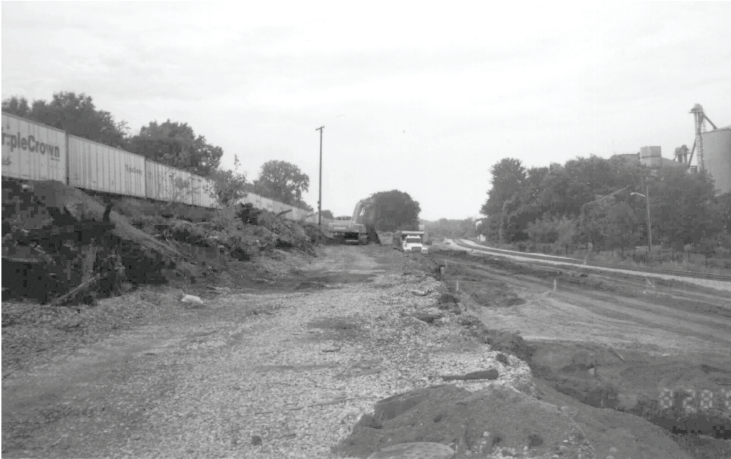
Figure 8-13. The site for mass excavation of a side slope in a rail yard incorporating a track excavator and dump trucks.
