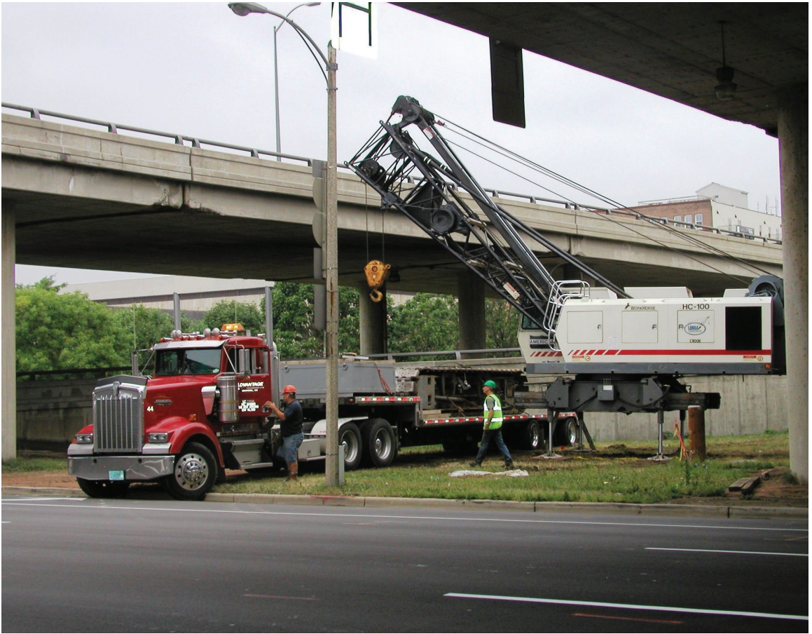
Figure 16-2. Demobilizing a crawler-mounted crane from the jobsite. As with mobilization, the costs incurred when demobilizing assets from the project can be substantial. The hauler rental and labor time for the pictured activity, plus the down time for the crane, can quickly cost thousands of dollars. Road movement permits may be required for oversized loads. All of these things must be planned—“spur of the moment” seldom suffices.
