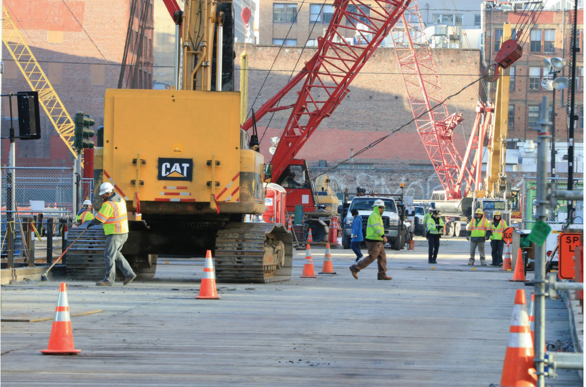
Figure 11-1. Examples of PPE worn at a construction site: Hard hats and vests are obvious.
