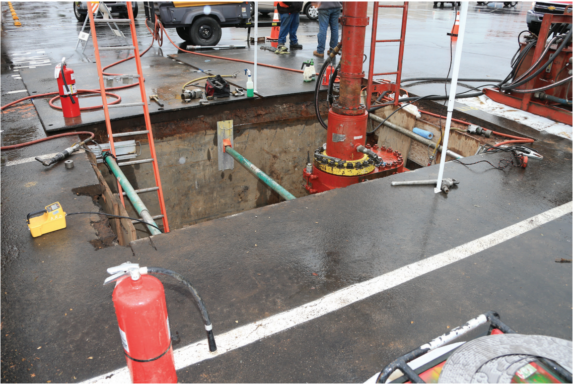
Figure 11-5. A shoring system installed for utility construction. Note that a barricade must be installed if the excavation is left unattended.
