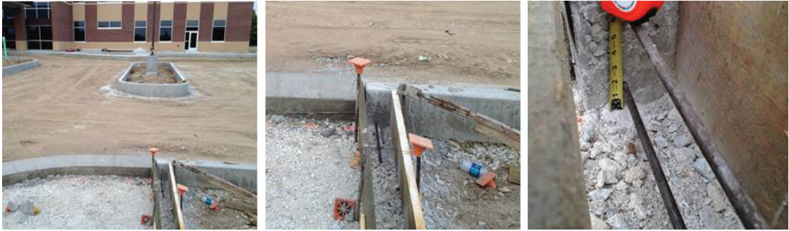
Figure 14-4. Curbing rebar photographs for nonconformance log, item number 4.
