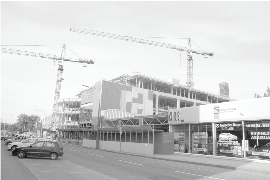
Figure 4-6. Typical hoarding: A solid perimeter barrier on a construction site in Ireland.
