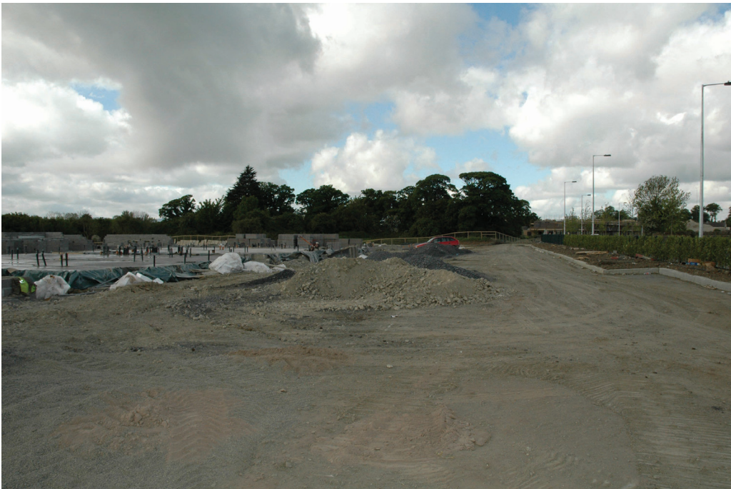
Figure 4-10. Temporary construction road layout built on the location of the future permanent roads.
