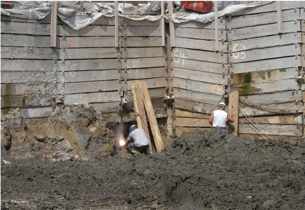
Figure 6-16. Welding bolts to hold wood lagging tightly to the driven H-piles. Encountering a layer of uncommonly plastic soil permits loads from the soil above to induce higher lateral pressures against the excavation supporting structure. Unexpected groundwater might also induce more pressure by increasing the weight of the soil mass while reducing its shear resistance. Not all subsurface conditions are discovered by common soil exploration procedures so builders must be observant.
