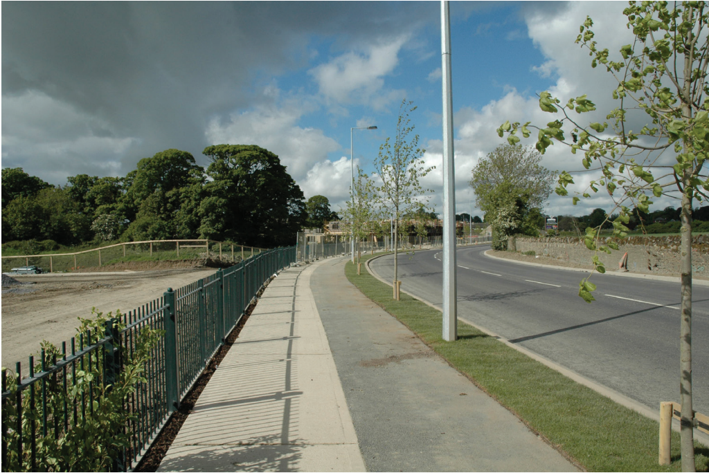
Figure 4-3. Assessing the nearby road network around the site for access into the site and material storage.
