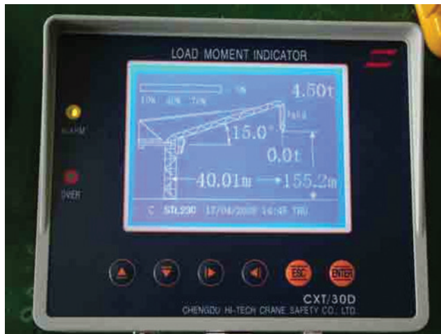
Figure 9-17. Hardware used to measure and display the real-time load moment on crane during operation. Source: Cranesmart.
