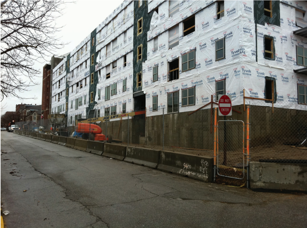
Figure 4-7. Typical fencing with concrete traffic bollards on a construction site in the United States.
