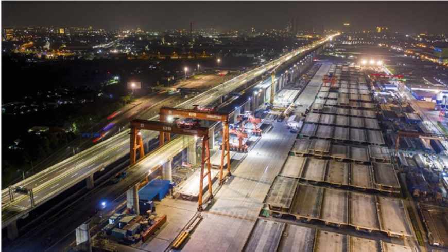
Fig. 2 Jakarta–Bandung HSR and Japek expressway are located side by side in this corridor section (Source Detik, 2021)
