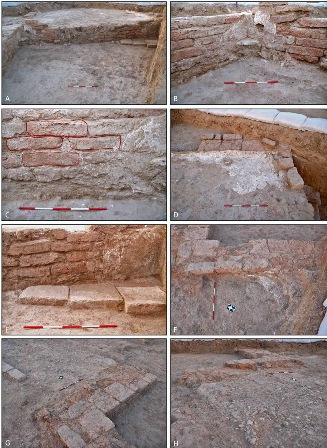
Figure 6.16 The baked brick structure in Area I: A) Room 1 (looking south), B) corner of Wall 4 and Wall 6, C) Wall 4 (looking northeast), D) corner of Wall 7 and Wall 6 in Room 3 with remnants of lime-plaster floor, E) paved floor in Room 1 (looking south), F) west face of Wall 3 with remnants of Room 4 lime-plaster floor, G) corner of Wall 3 and Wall 9 and part of Wall 10 with pebbled courtyard to the north, H) pebbled courtyard (looking south).
