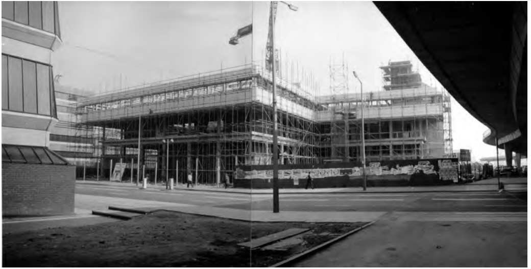
Figure 2.32 NCC under construction. The shadow of Mancunian Way fills the frame on the right. The left foreground is the edge of the John Dalton Building, and in the background is the BBC.
