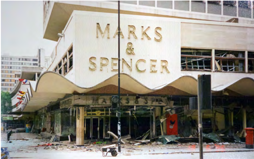
Figure 5.01 Cross Street Manchester, 15 June 1996. The wavy canopy of Marks & Spencer was partially destroyed at the epicenter of the blast. Also visible is the Portland stone cladding.
