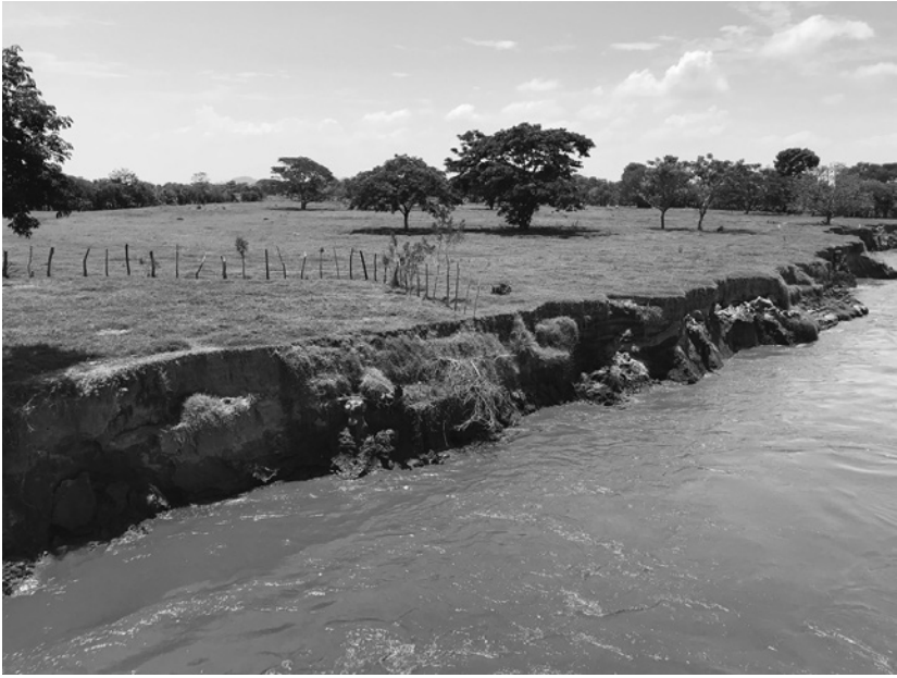
FIGURE 3.3. Embankment allegedly damaged by riverboat traffic, Pinillos, Bolívar. Source: photograph by author.
