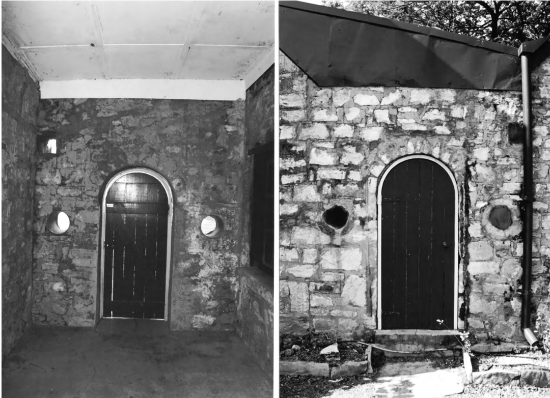
Figure 10.10. Interior (left) and exterior (right) of the circular embrasures either side of the rear door of Springvale homestead.
