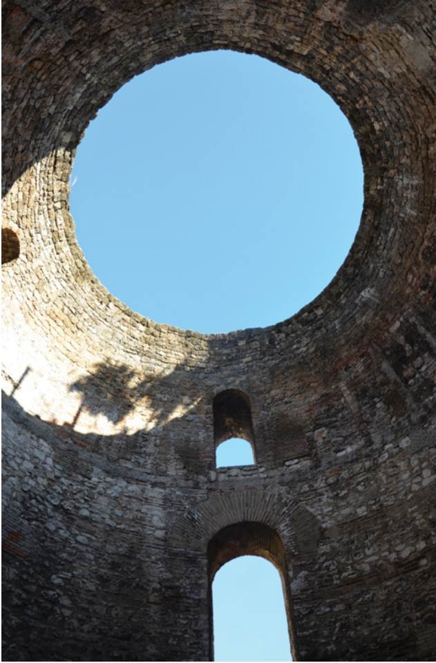
FIGURE 11.11 Domed roof of the 'Throne Room,' Diocletian's palace, Split. Executed in pitched brick technique.
