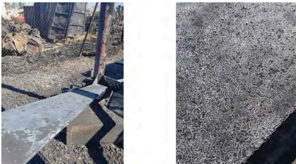
Figure 7. The blue temper on bracing sections in the bottom segment of the tower.
