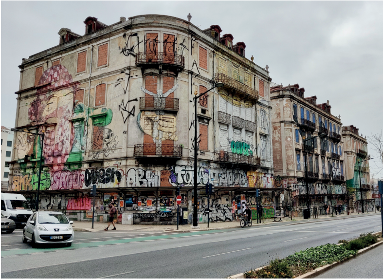
Figure 3.8 Heritage issues can trump other design factors, including in a redevelopment scheme for three empty buildings in Lisbon city centre on the Avenue Fontes Pereira de Melo. While the redevelopment of these buildings was designed by Souto Moura, a Pritzker-winning architect, the scheme was rejected by the municipality after receiving a negative review from the Ministry's advisory body (image: João Bento).
