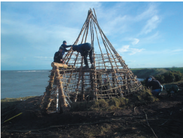
Figure 13.10 The hut begins to take shape as an entrance is attached and the turfing begins.
