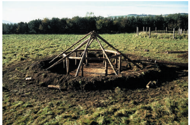
Figure 13.3 The hut after erection of the timber uprights, lintels and roofing poles
