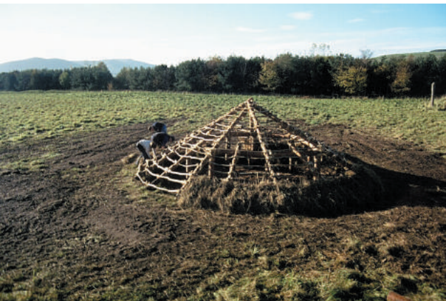
Figure 13.5 Adding the first layer of thatch starting from the base of the roof.
