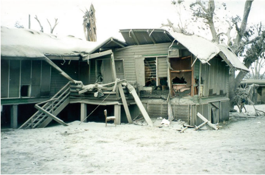
Fig. 4 A Rabaul (Papua New Guinea) suburban house severely damaged (total loss) by 600–800 mm ash fall from Tavurvur volcano in 1994. The timber-framed roof has collapsed inwards and the walls spread outwards. The sub-floor area has been buried by air fall ash and minor lahars (Photo R Blong)
