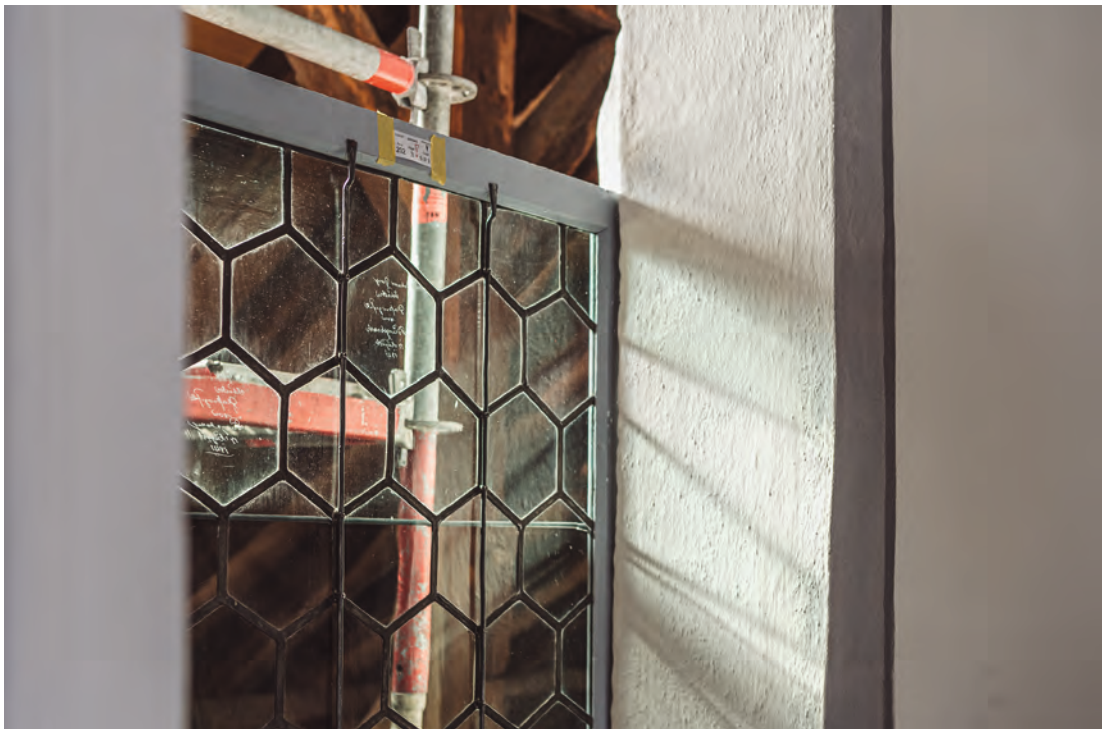
6 Crown glass used for the hexagonal glazing on the south side of the choir of St Michael's, Bamberg.
