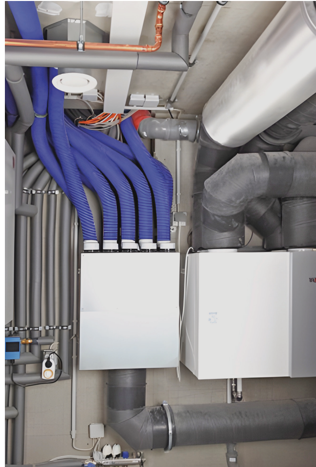
Figure 11.14 Image of whole house ventilation system with HRV. 4
