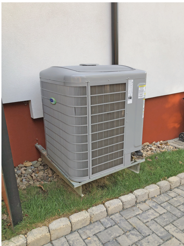
Figure 11.6 Large whole building heat pump.
