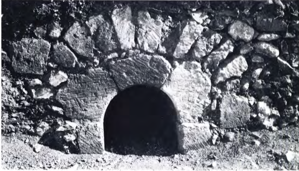
a. The arch, possibly a drain or water channel, in the south-east corner of the salsary (4k)
