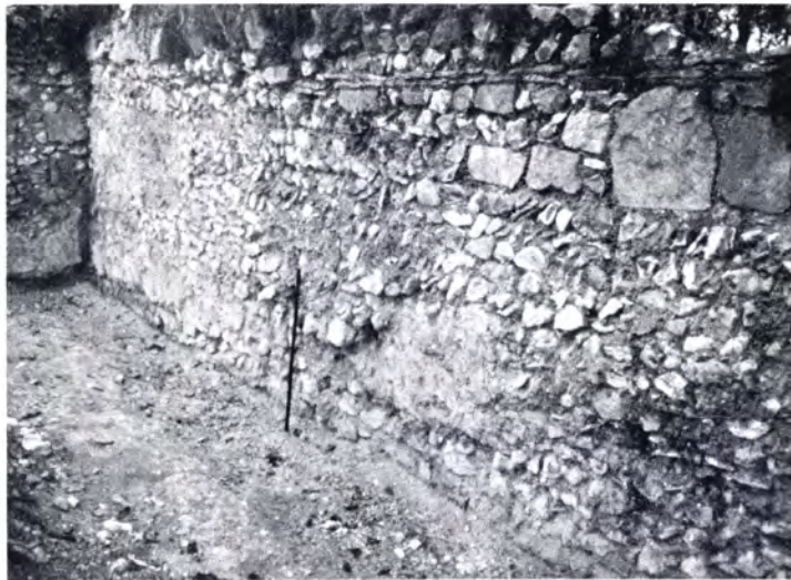
b. The west wall of the herlebecheria (4f), showing what was described in the 1930s as 'Edwardian rebuilding'. Note two-foot rule against the wall
