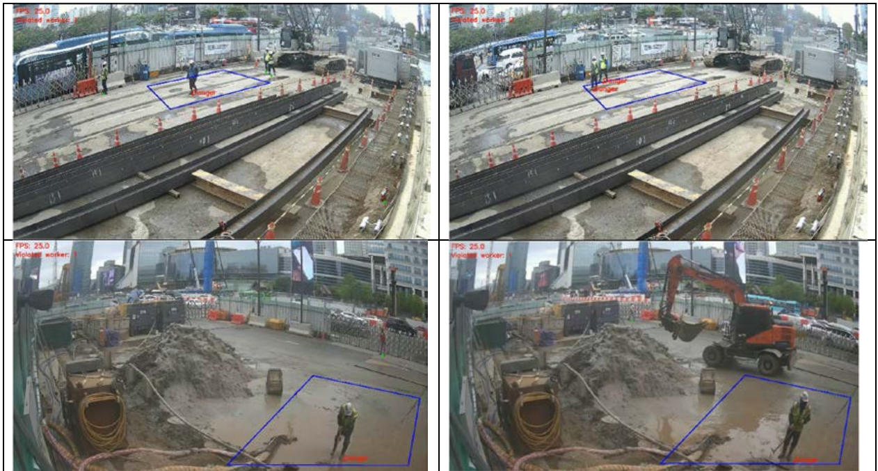
Figure 5. Detect workers in the danger area
