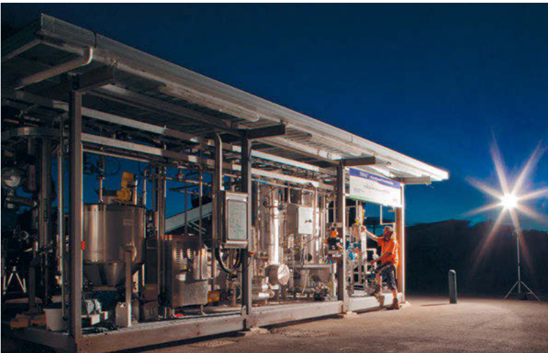
Fig. 13.4 TERAX pilot plant, Rotorua District Council's Wastewater Treatment Plant
