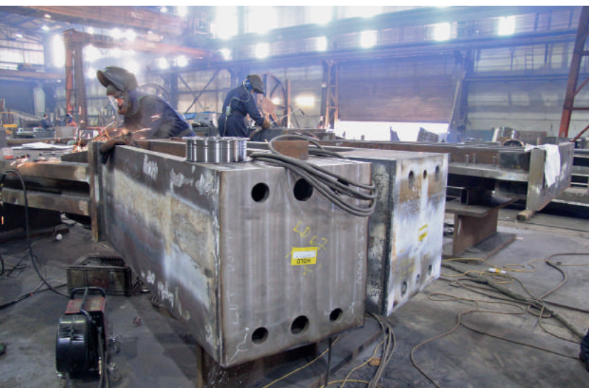
Fig. 12: Subassembly in finishing pass with robotic milled endplates. After the welding process, the complete node is offered up to a multi-axis milling robot and endplates are machined to exactly match the fabrication model. This eliminates the tolerances introduced by geometric distortions caused by induced heat.
