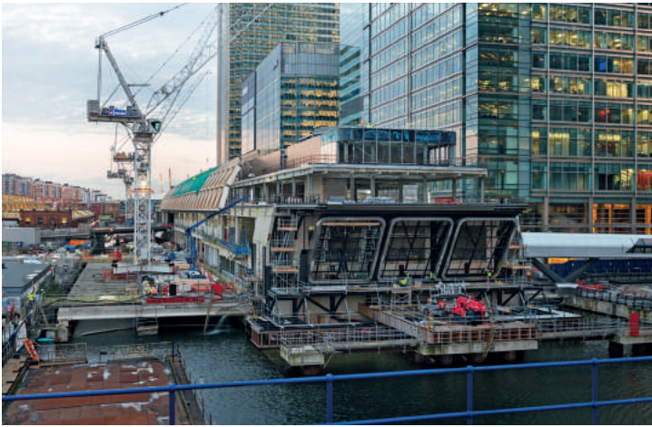
Fig. 3: Photograph of site showing construction progress mid-November 2013. The photograph shows the concrete substructure with end pavilion steelwork, station extractor cladding and the timber beams in the central section installed. (Photo: Nigel Young / Foster + Partners.)
