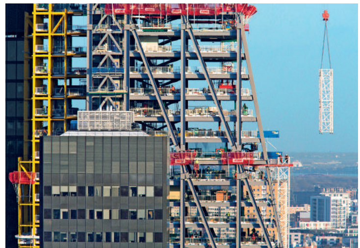
Fig. 2: Lifting operations take place 24/7. Most large elements are assembled during the night shift, as day traffic does not allow delivery of the 27 m long columns. Due to the high degree of prefabrication, the superstructure was erected in 16 months. The first superstructure elements arrived on site in January 2012.
