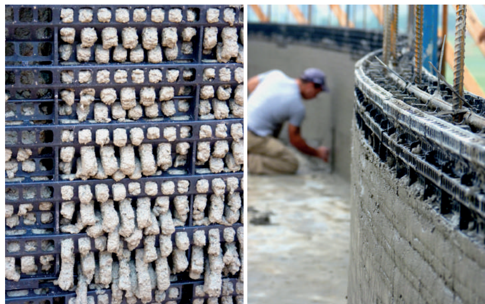
Fig. 2: Leaking formwork by Forma-Tech. (Image by courtesy of Forma-Tech International.)
