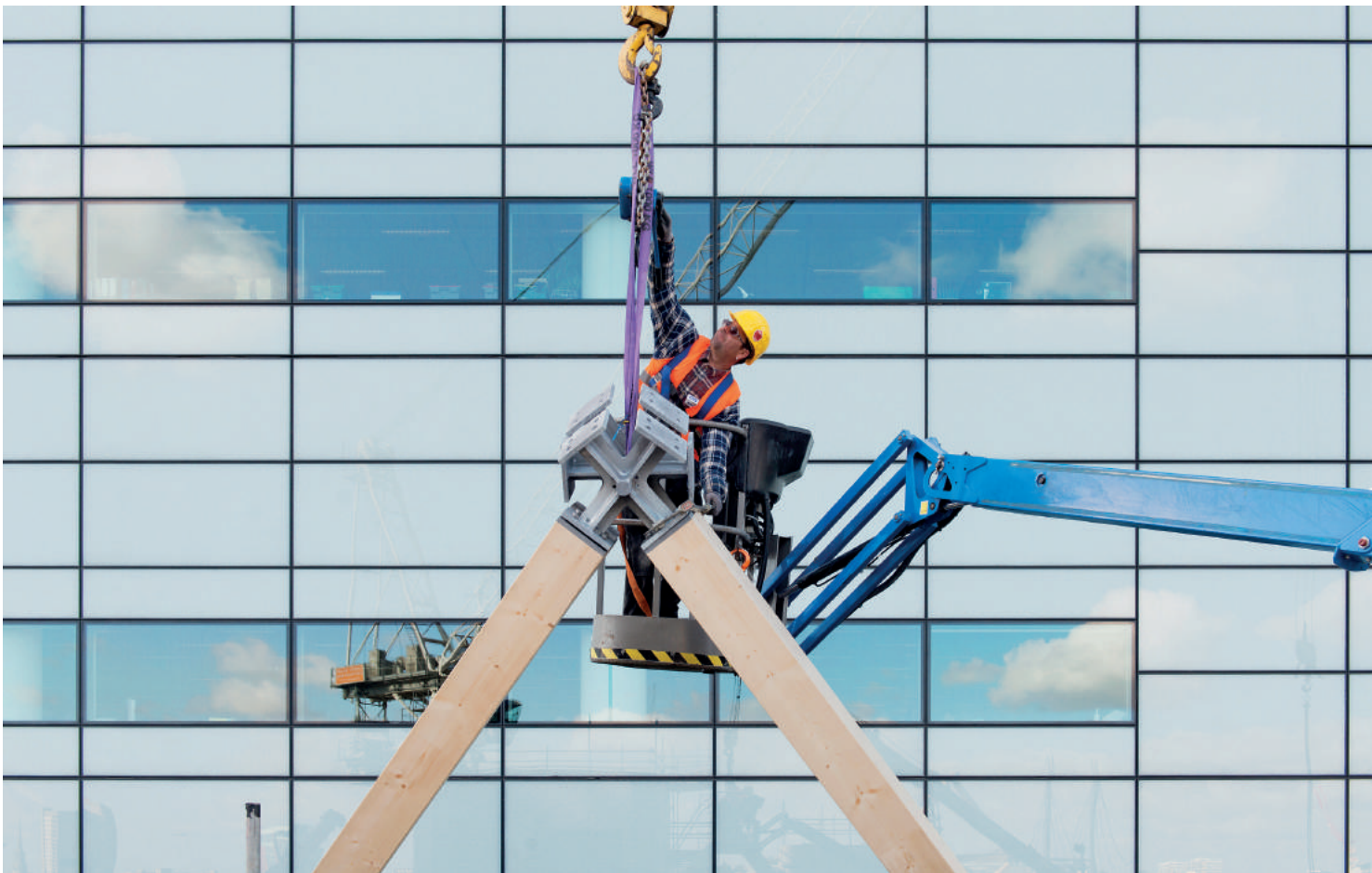
Fig. 10: Photograph capturing on-site installation process for nodes using crane and cherry picker. (Photo: Nigel Young / Foster + Partners.)
