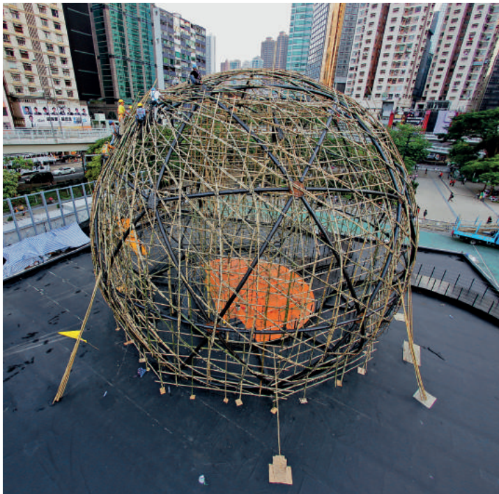
Fig. 5: Installation of secondary bamboo substructure. (Photo: Laboratory for Explorative Architecture & Design Ltd.)
