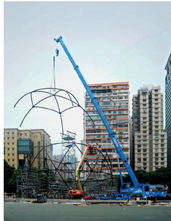
Fig. 3: Installation of geodesic steel dome structure. (Photo: Laboratory for Explorative Architecture & Design Ltd.)
