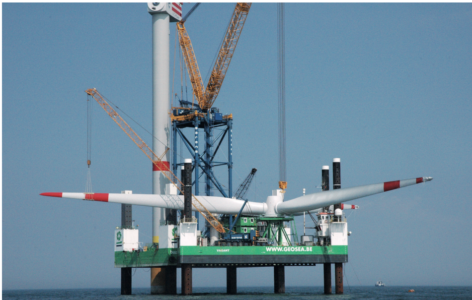
■ Photo 11 : blade (126 m in diameter) being mounted on the mast in the 300 MW Thornton bank offshore wind farm in Belgium (© Deme, BE).
