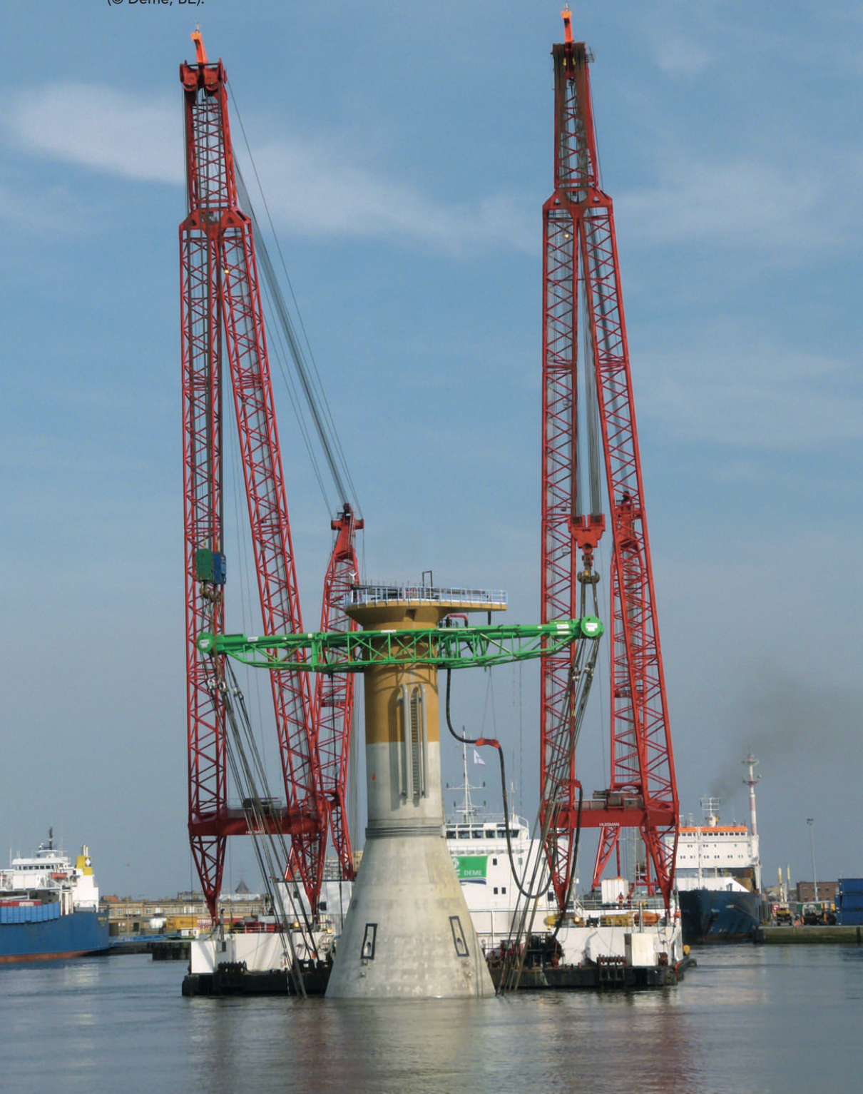
Photo 17 : transporting the foundation for a 5 MW offshore wind turbine on Thornton Bank (© Deme, BE).
