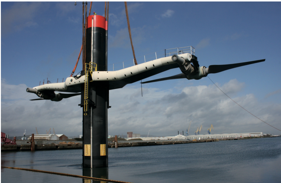
■ Photo 30 : Seagen stream turbine installed at Strangford Narrows in Northern Ireland (© Marine Current Turbines Ltd, UK).
