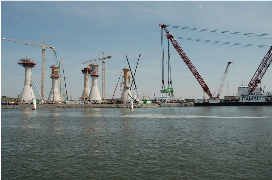
■ Photo 35 : construction site for the foundations of the 300 MW Thornton Bank offshore wind farm in Belgium (© Deme, BE).
