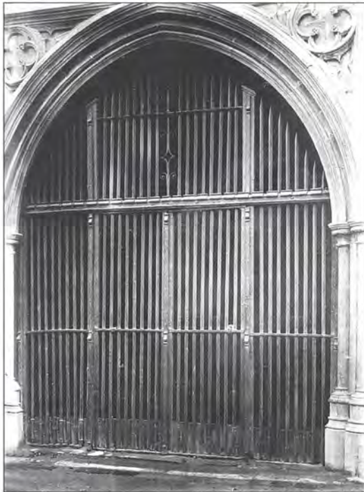
6.125 Canterbury Cathedral, grille from nave, now in west porch (photograph: © Crown Copyright, RCHME).
