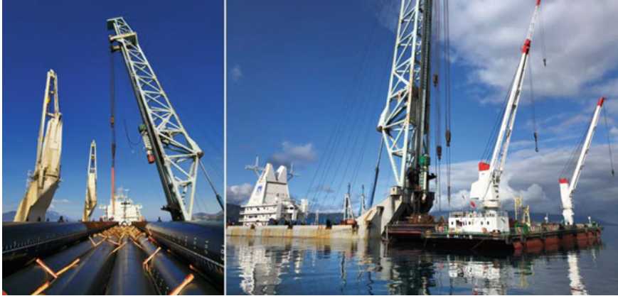
Fig. 4.11 Construction of steel pipes (Left: steel pipe transportation; Right: steel pipe welding)
