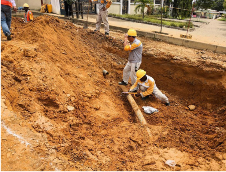
Fig. 3.8 The CRCC is helping local government organs repair damaged water supply pipelines
