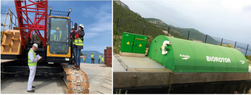
Fig. 4.14 Third-party inspection of the construction equipment and domestic sewage treatment system in the living quarter
