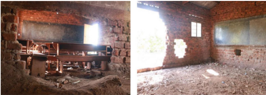
Fig. 9.17 Nakakandwa RC primary school before the repair
