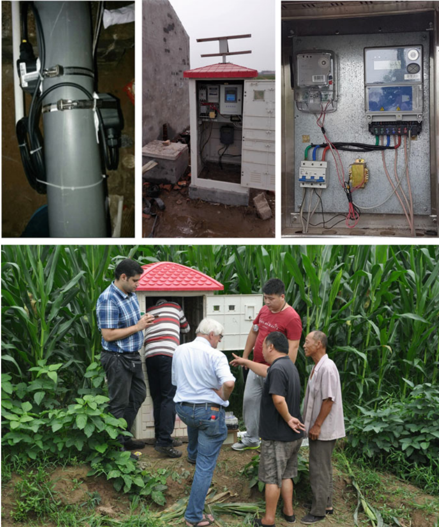
Fig. 4.14 Hengyuan meter and RSA meter. Upper left: The Hengyuan ultrasonic water meter; Upper middle: The meter is protected by a concrete box. The control box and data transmission unit are protected by a plastic hut; Upper right: RSA meter box; Bottom: Swiss expert answering questions from the local farmers during the installation of RSA meters by technicians from RSA and local DWR
