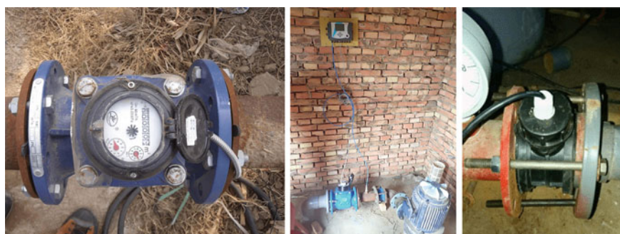
Fig. 4.13 The Hengze meter (left), the Itron meter with transmission unit Watermind on the wall (middle) and the Haisen meter (right)
