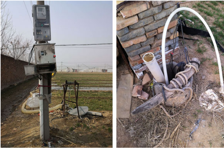
Fig. 4.12 Typical irrigation wells and electricity meters installed in Guantao County
