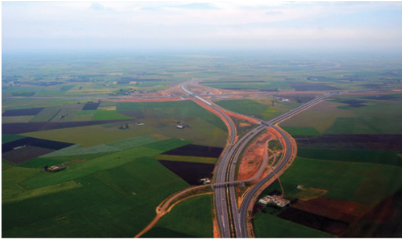
Figure AW1.2: New highway construction in Casablanca: how will the promises of infrastructure be justified?
