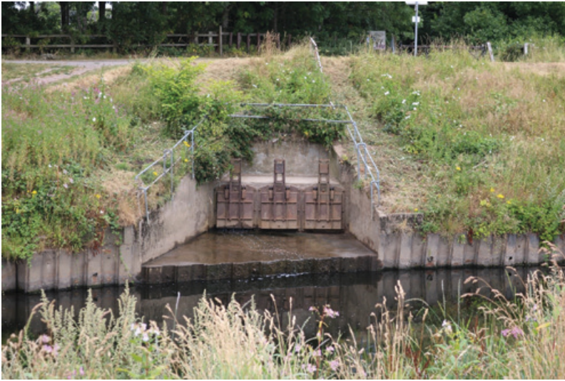
Figure 6.2: Bradley Lane combined sewer overflow, flowing into the River Mersey, Stretford, Trafford, Greater Manchester
