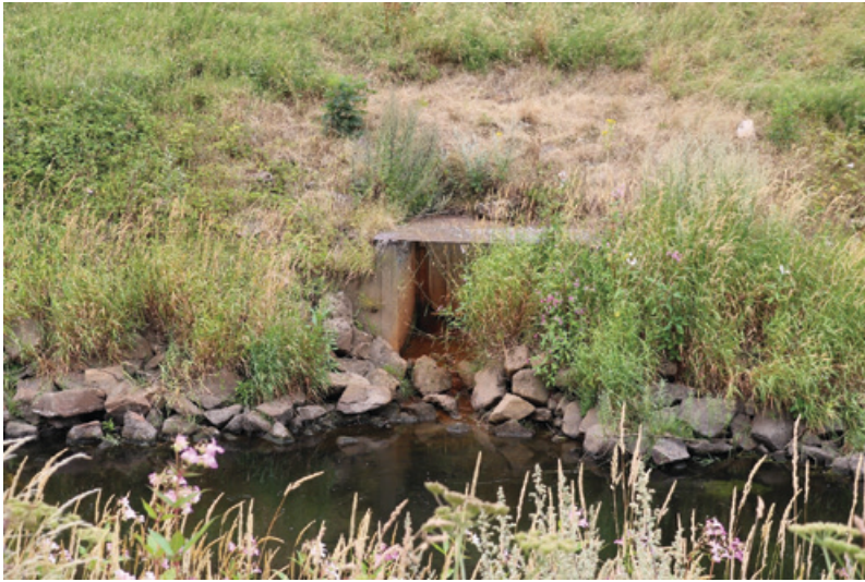
Figure 6.1: Walwyn Close combined sewer overflow, flowing into the River Mersey, Stretford, Trafford, Greater Manchester
